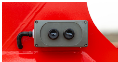
Walk along gate control located on the hopper sidewall
